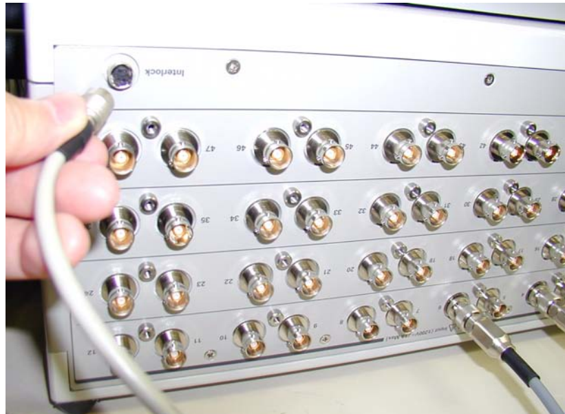
Interlock Cable Connection on Agilent B2220A
